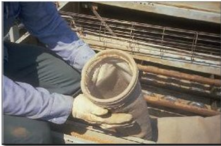
Pulse Jet Baghouse for Particulate Removal
